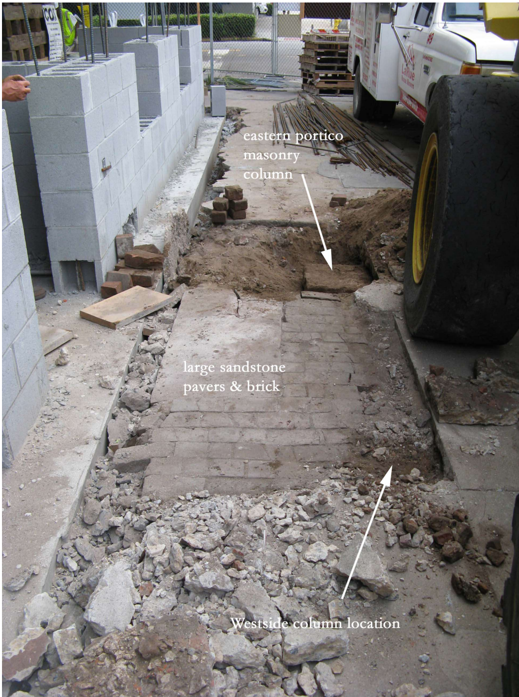
View of the sidewalk excavation for the front portico. The square pad matches exactly the size and location of eastern masonry column of our proposed design.
