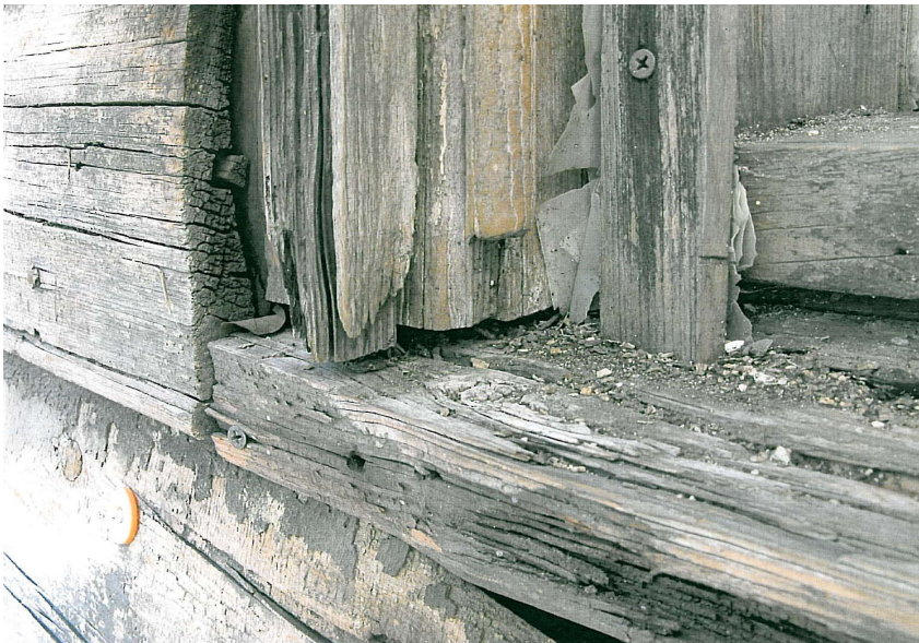
Typical window condition for the building . Window are to be replaced with approved TDL DH by Kolbe.
