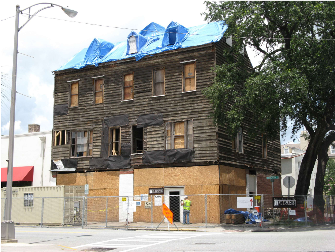
Broughton Street elevation before after stucco removal and before lowering in July 2013
