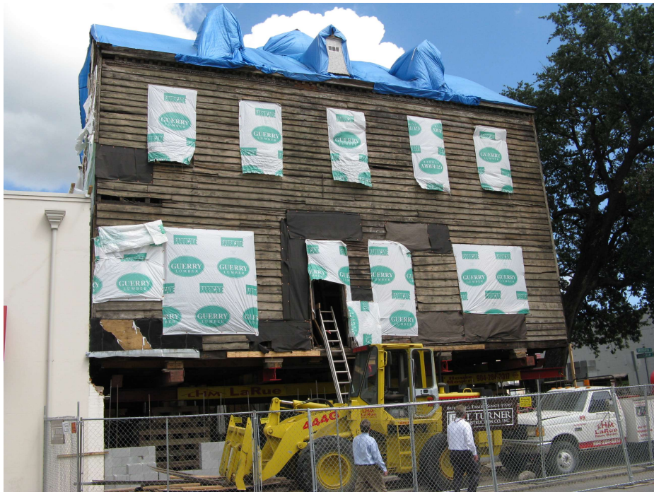
Berrien House as of 9-18-2013 . Perimeter wall 75% complete, repairs between Blick building complete and building lowered 2' of the 3'8''.
