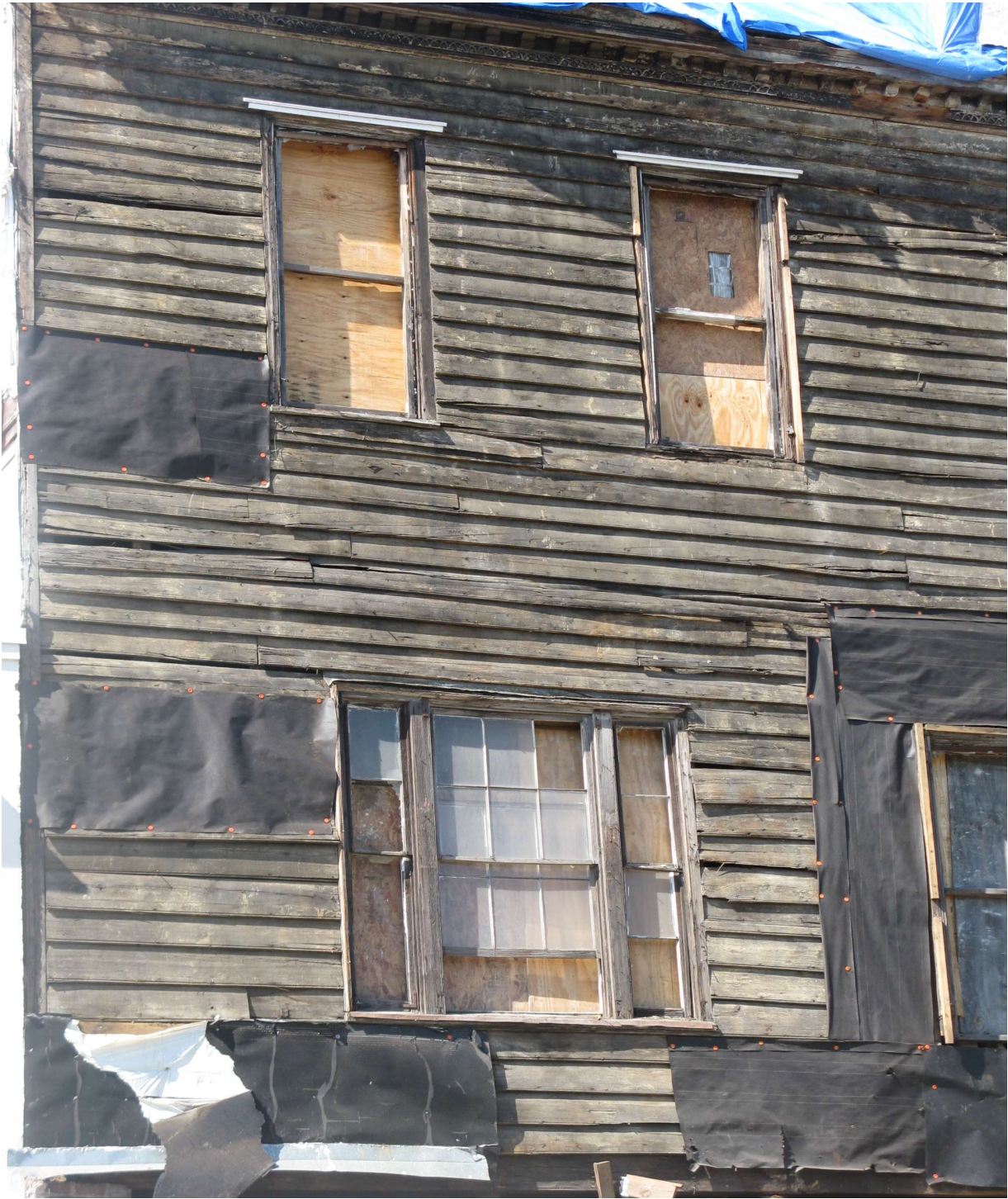
Closer view of front facade after stucco removal show the poor condition of siding and windows.
