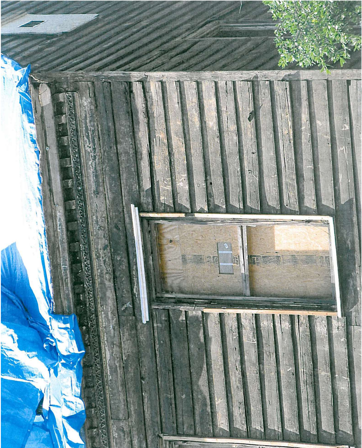
Removal of the stucco revealed the original cornice is good condition. Water damage will require replication of some of the details.
