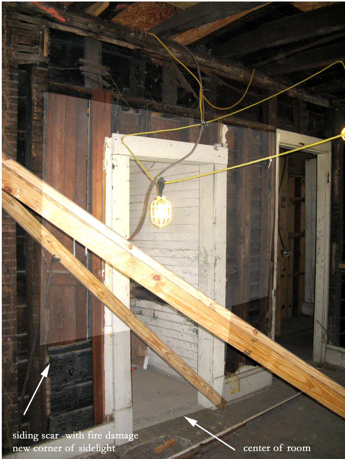
West side shed addition looking north. Show the same cut in the siding as the east side room. Here you can see the fire damage on the back of the siding. The highlighted area shows restored french
