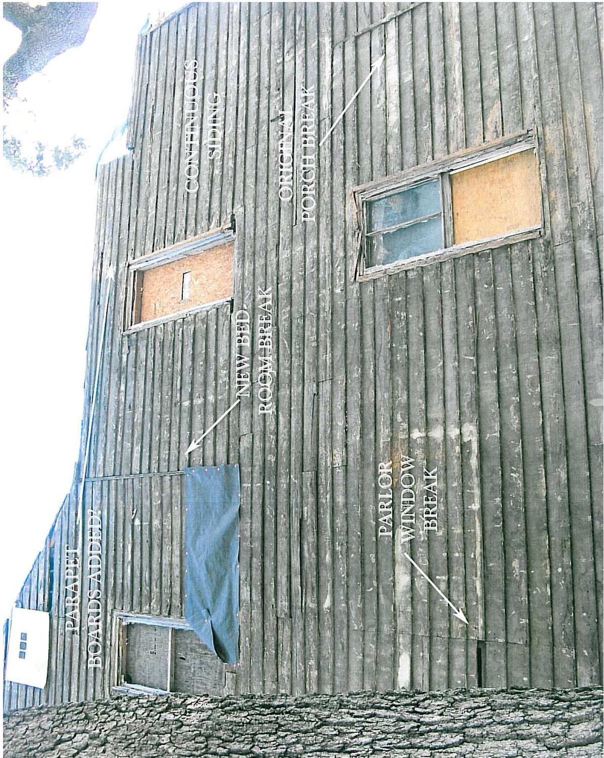
Habersham elevation shows the evolution of the building in the breaks of the siding . The third floor rear shed rooms and sleeping porches were added c.1830-1840 by John Macpherson Berrien.
