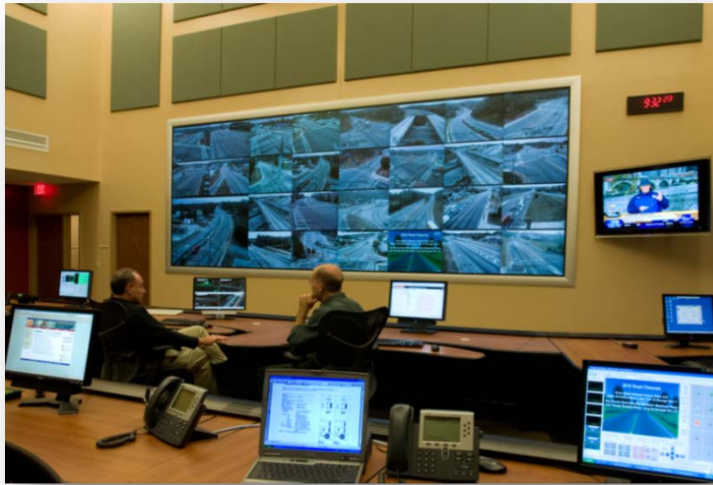
Figure 10-2: Cobb County Traffic Management Center
