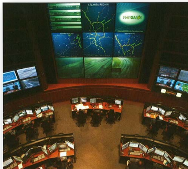
Figure 10-3: Control Room in the GDOT TMC
