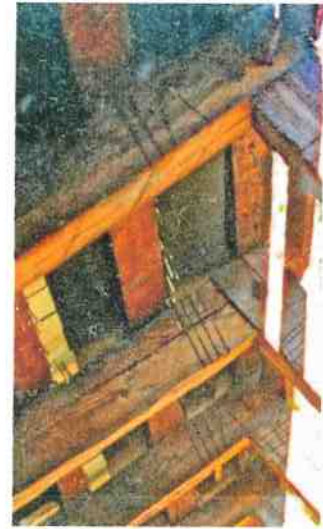
Figure 3. Hewn & pit sawn rafters. Apex mortise, tenon, and pegged joint. Note the carpenters' layout marks. Photo c. 1997, Arndt Family.
