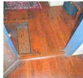
Figure 9. Break joint in floorboards in the garret on north side of the stair well.
