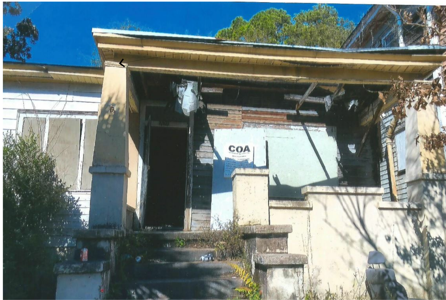
PHOTO OF ORIGINAL DAMAGED FRONT PORCH (3)
