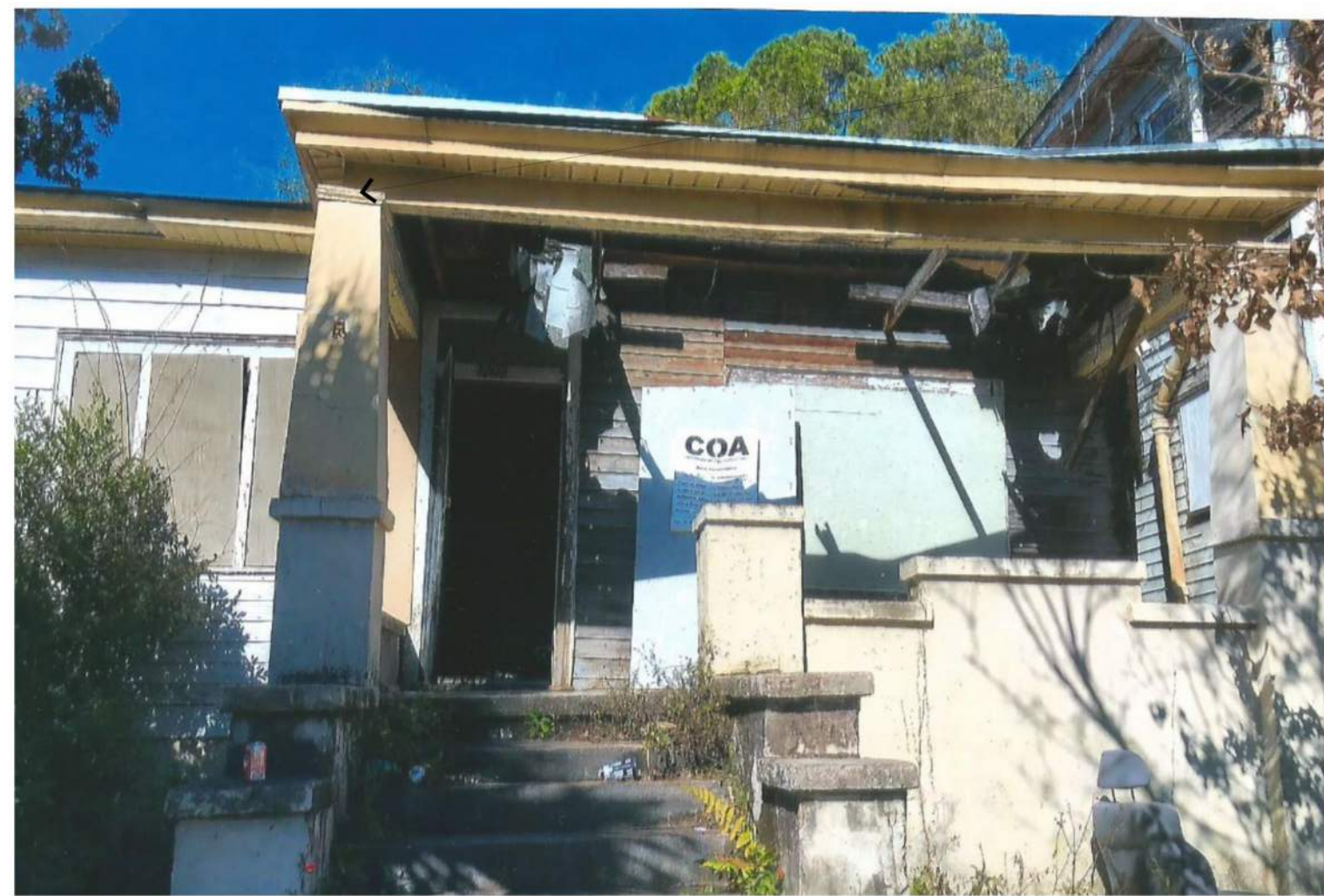
PHOTO POST-FIRE ORIGINAL DAMAGED FRONT PORCH 3
