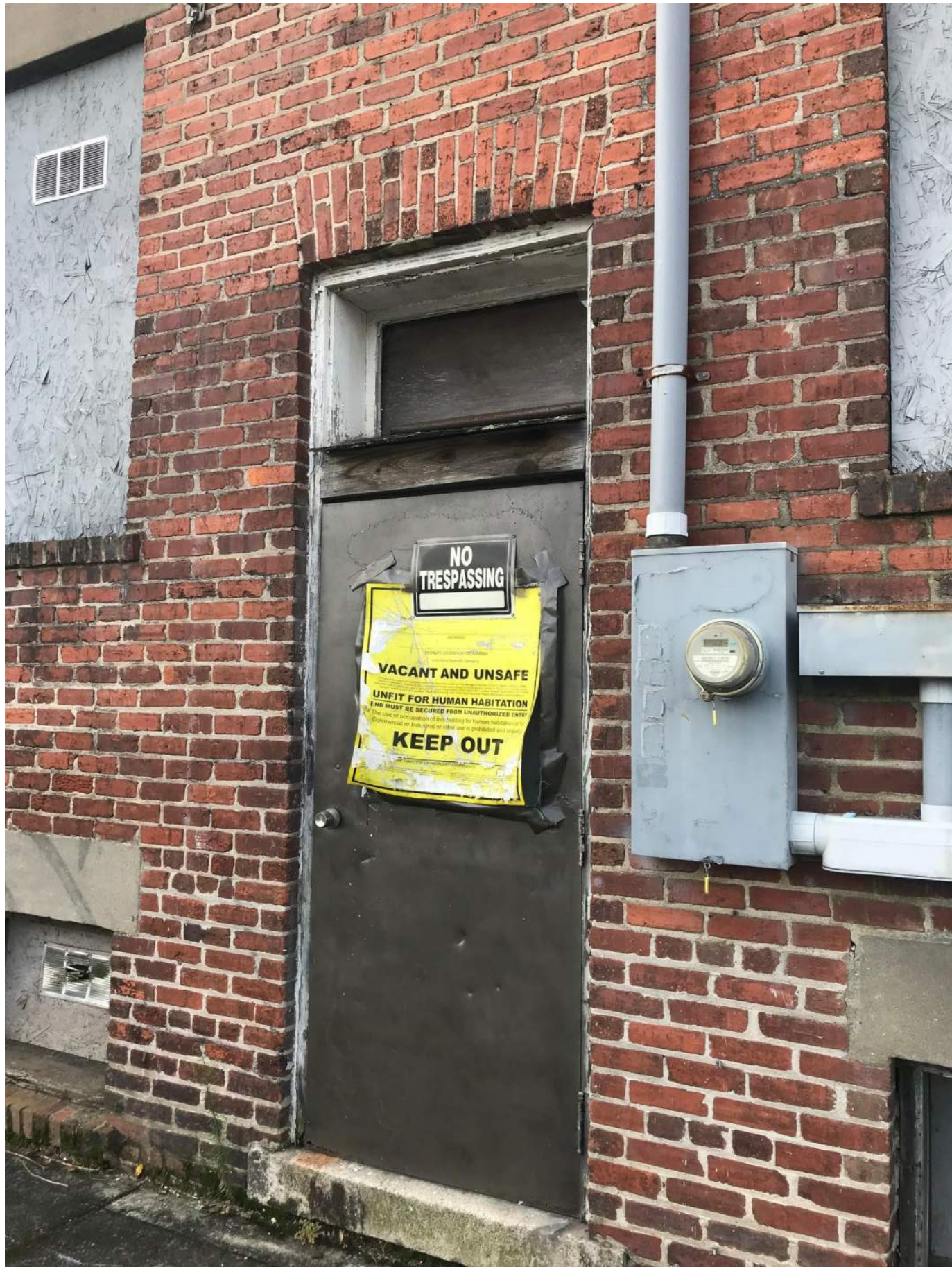
NOTE: REAR DOOR REPLACED WITH H.M. AT SOME POINT
