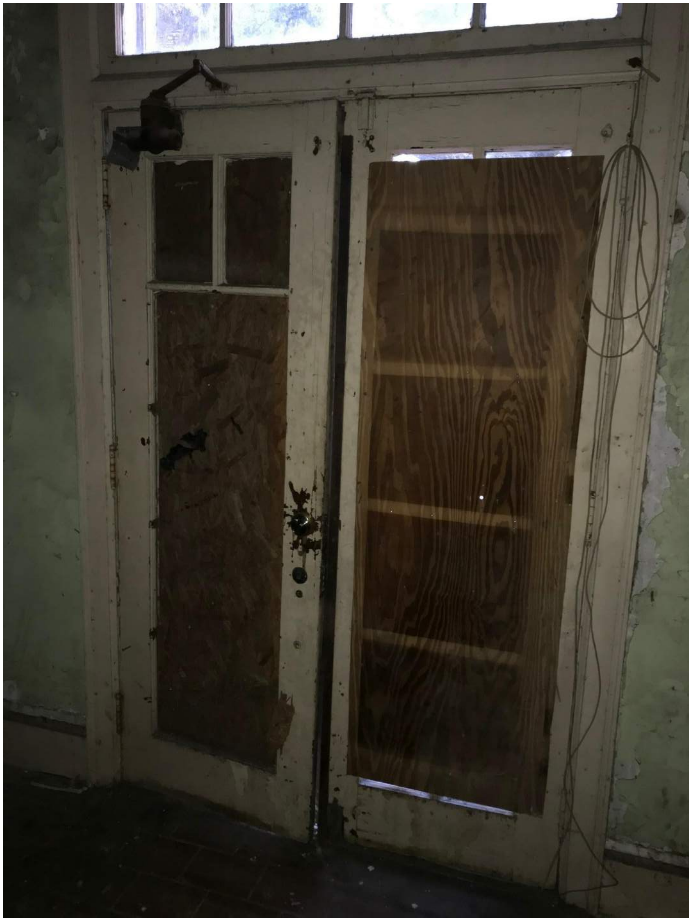
NOTE: MISSING DIVIDERS AND GLASS
