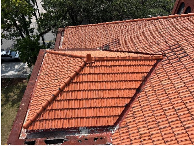
Built-in gutters deteriorated, Previous repair attempts with asphalt mastic on tiles
