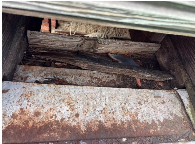
Built-in gutter deteriorated, interior visible from the roof
