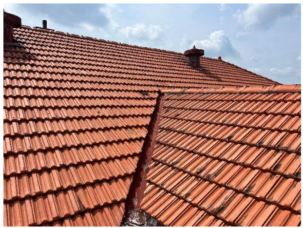
Deteriorated metal valleys
