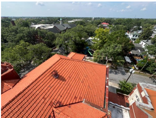
Damaged tiles, multiple previous repair attempts
