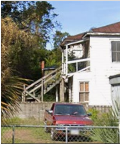
View from West 40 th Street and the current condition of the rear porch and stairs.
