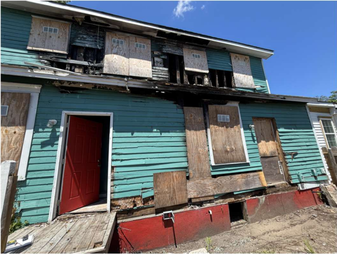
SOUTH ELEVATION FIRE DAMAGE
