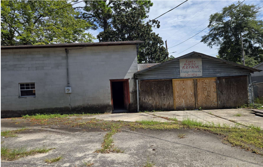
Photo 1: View of CMU block auto repair structure and detached garage (Lewis Auto Repair) — boarded bays, structural deterioration, and overgrown site conditions evident.
