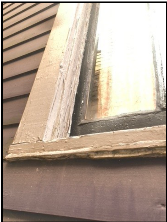
Example of deteriorated trim. To be replaced.
