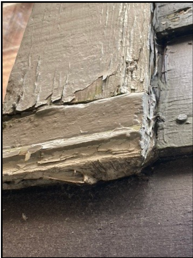
Example of deteriorated trim. To be replaced.
