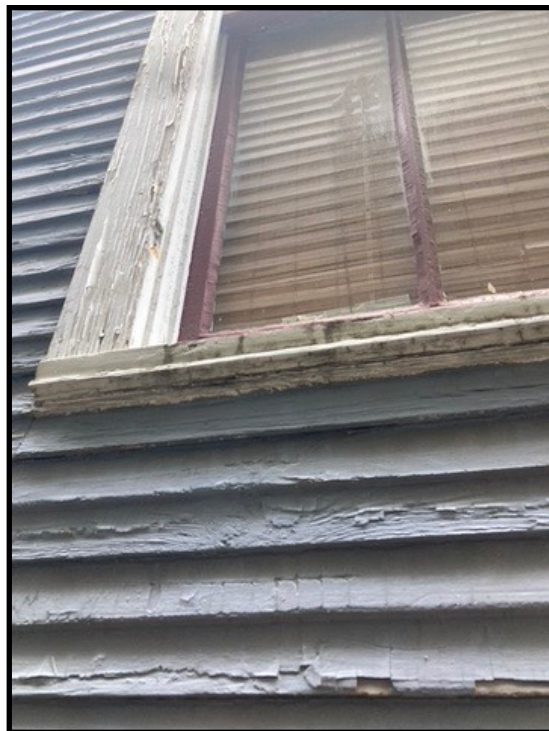
Example of deteriorated trim and siding. To be replaced.
