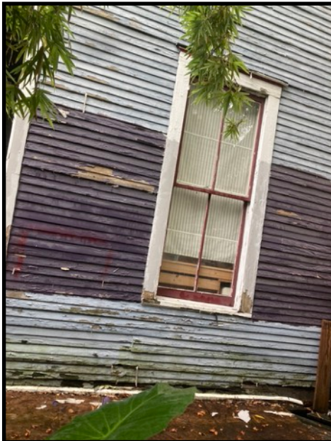
Rear side of house, forward section. All siding and trim to be replaced.
