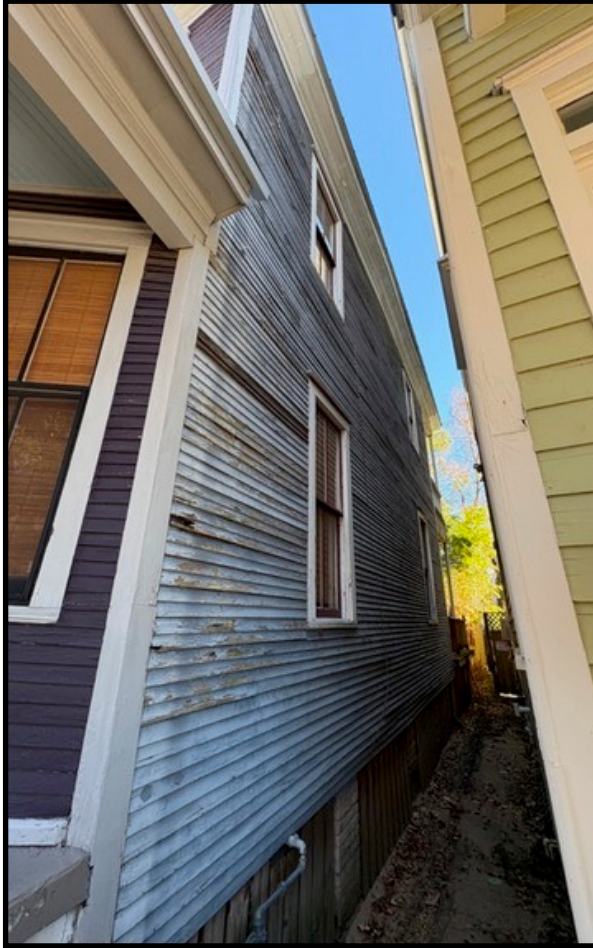
South side of house, full view. Siding on this side to be replaced in full.
