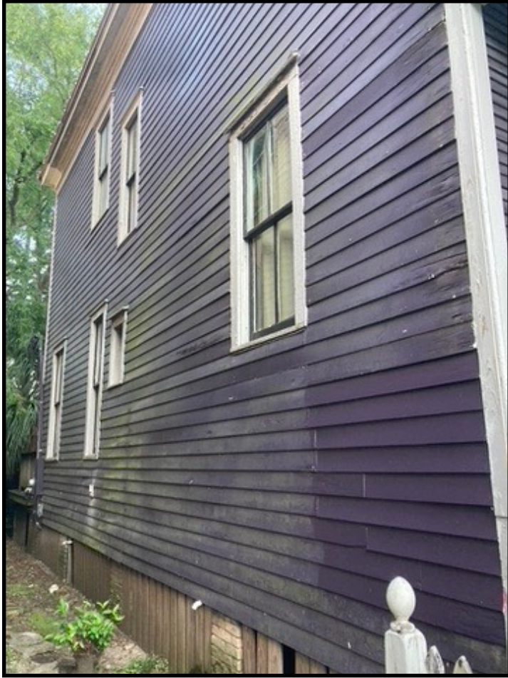
North side of house. Siding not consistent with original. To be replaced.
