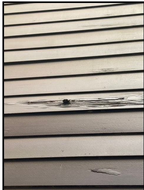
Example of damage on north side, typical of moderate damage on that side.
