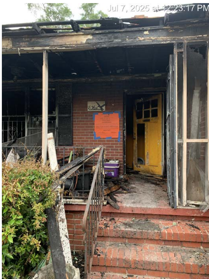
3. Damage after fire
