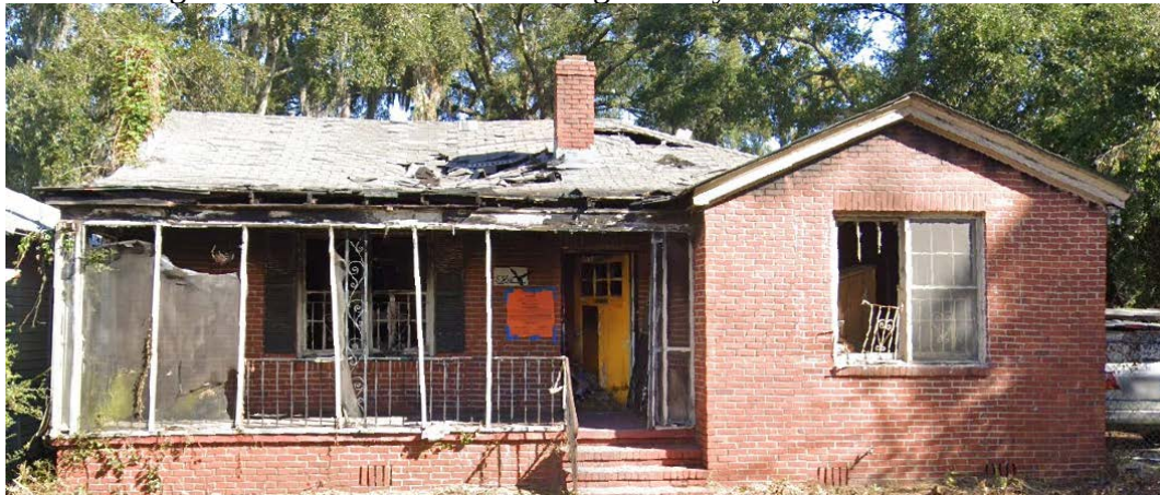
1. Roof and column damage after fire
