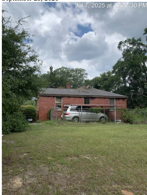
2. Damage after fire
