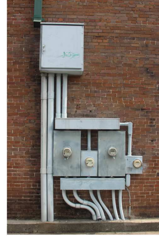
EXISTING ELECTRIC SERVICE
