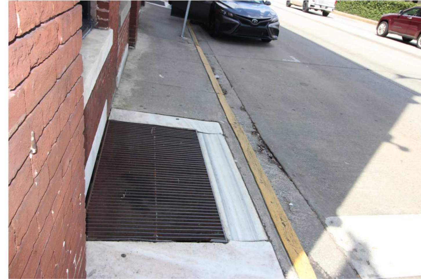
PROPOSE WIDENING OF EXISTING SIDEWALK TO CITY OF SAVANNAH REPLACE EXISTING SIDEWALK GRATING
