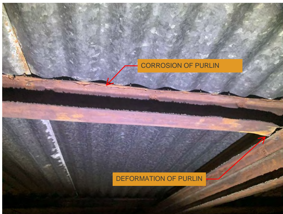
Photo 5: Purlins – Mild corrosion
