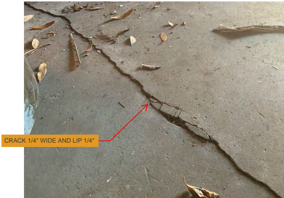
Photo 13: Ground Slab - Cracking
