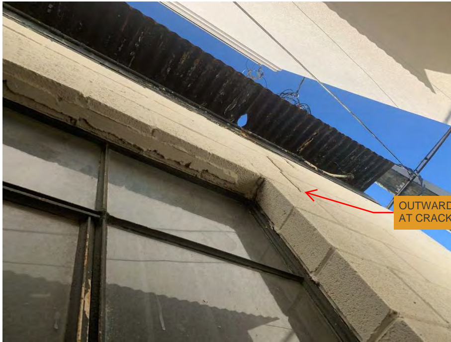
Photo 12: Exterior Wall – Cracking/shifting
