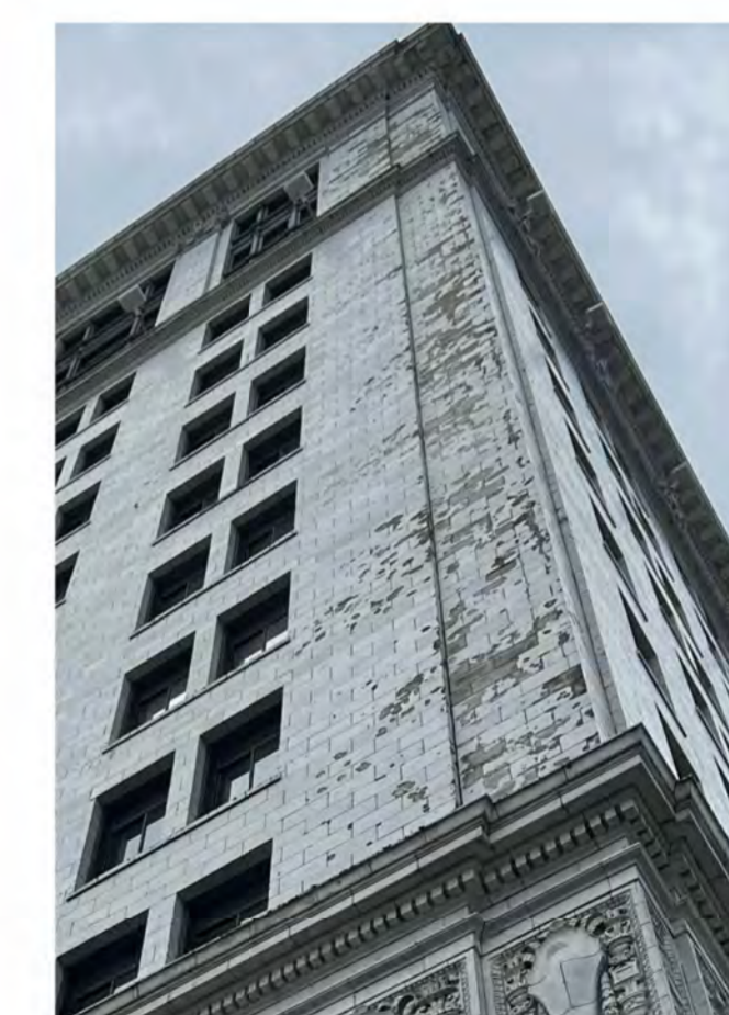
04- EXISTING EXTERIOR TILE TO BE REPAIR
