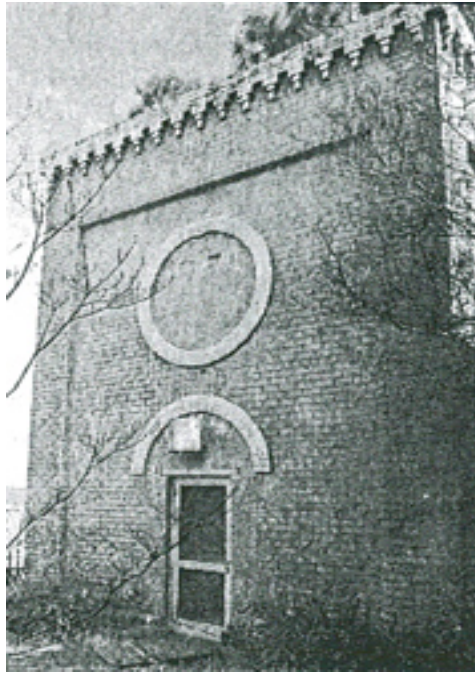
Above: photograph of the Tower Building /Exhausting Engine Building that collapsed during the clean up.
