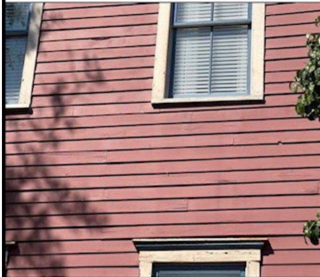
Item 10(Picture) Repair/replace/seal damage siding/trim to maintain integrity of the building's envelope.
