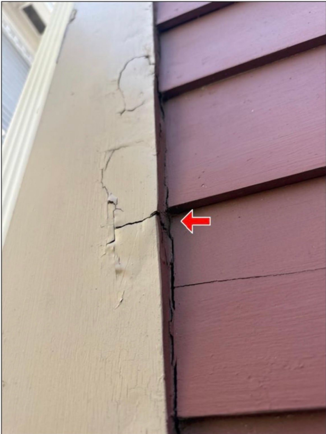
2.0 Item 2(Picture) Repair/replace/seal damage siding to maintain the integrity of the building's envelope
