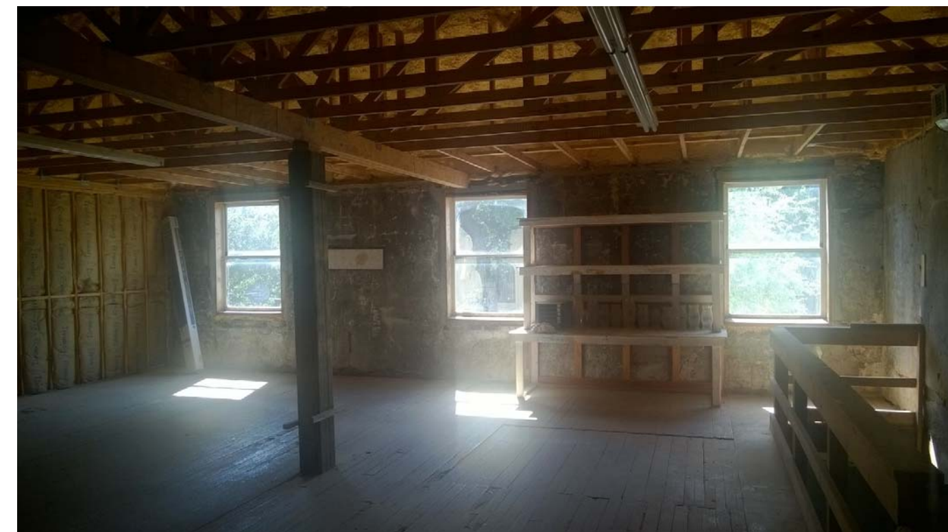
D. SECOND FLOOR, MLK BLVD SIDE, WEST WALL. NOTE BEAM AT WINDOW HEADER INDICATES NON-HISTORIC WINDOW OPENINGS. REFERENCE STRUCTURAL REPORT ITEM 3, PAGE 2 OF 14.
