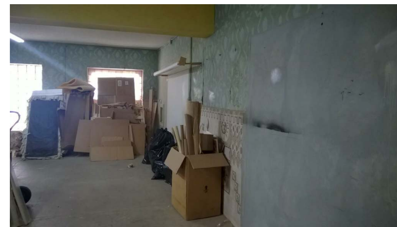
J. FIRST FLOOR, VIEW SOUTHWEST, INFILLED OPENINGS VISIBLE ALONG MLK JR. BLVD
