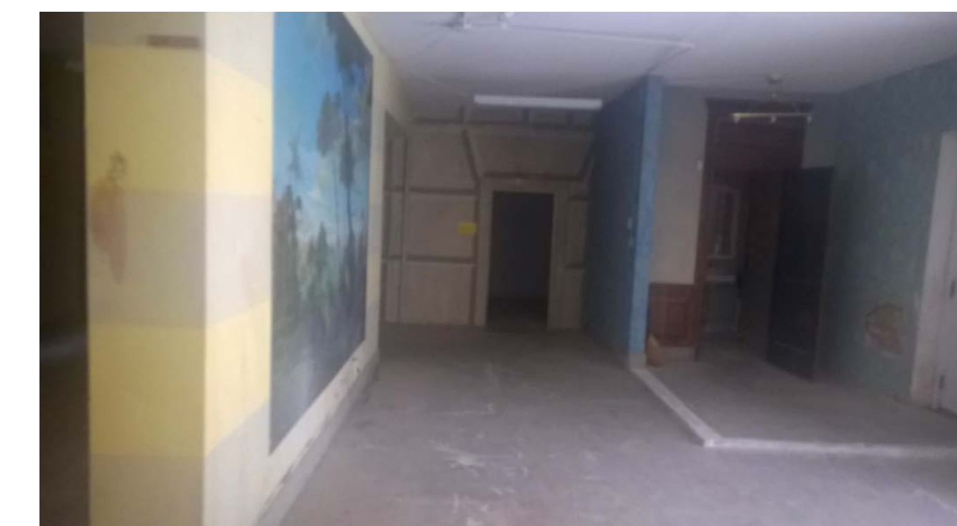
H. FIRST FLOOR, VIEW EAST TOWARDS CONCEALED MASONRY WALL, ASSUMED TO BE HISTORIC BUILDING EXTERIOR WALL
