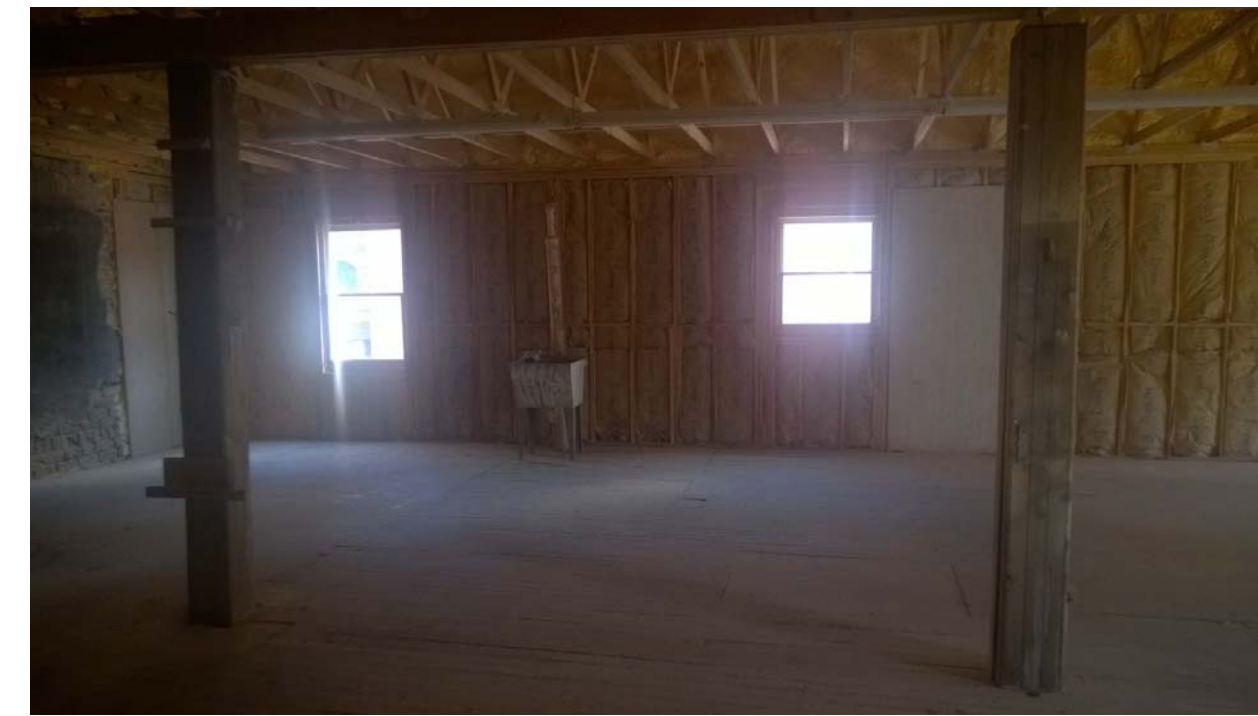
B. SECOND FLOOR, NEW CONSTRUCTION ENTIRE SOUTH WALL & ROOF STRUCTURE. NOTE OPENING PROPORTIONS WITH INCONSISTENT RYTHEM AND CHANGE IN FLOORING MATERIAL INDICATES ASSUMED LINE OF ORIGINAL BUILDING EXTERIOR.
