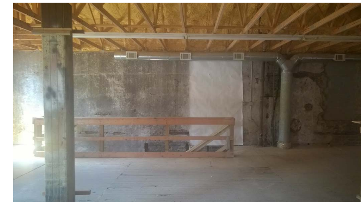
E. SECOND FLOOR, NORTH WALL (ADJACENT TO 30 MLK); NOTE NOTCHES IN MASORNY INDICATE PREVIOUS FLOOR SYSTEM EXISTED; NON-HISTORIC STAIR.
