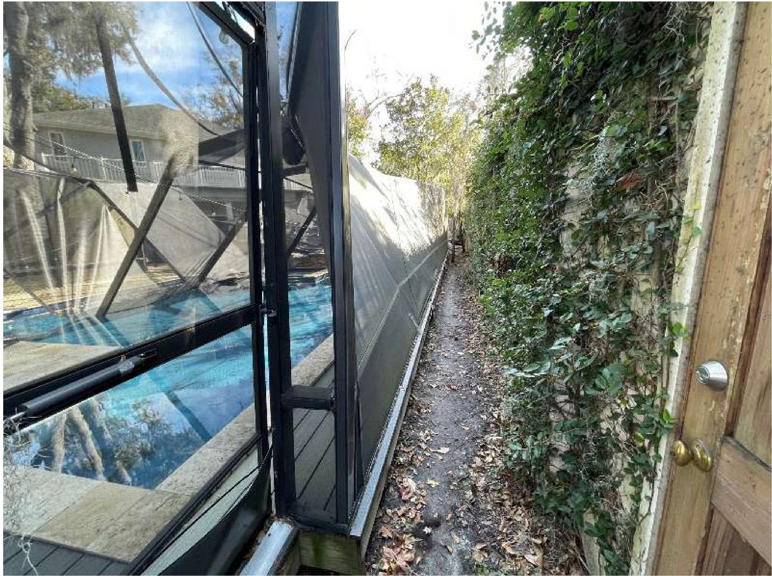
3 PH1.1 EXISTING ENCLOSURE DAMAGE SOUTH IMAGE 1/4" = 1'-0"
