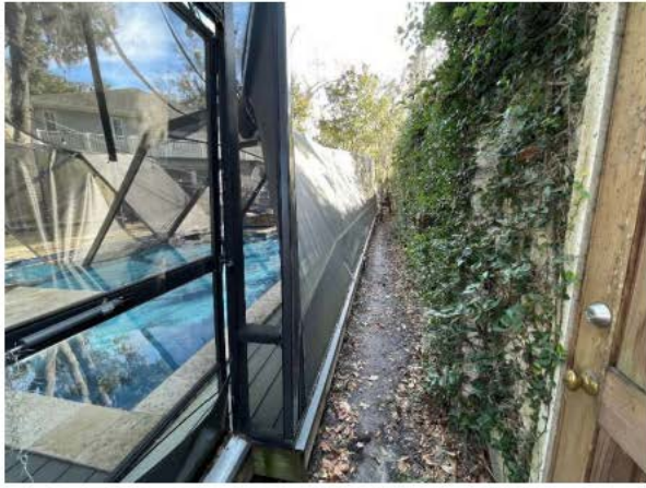
EXISTING ENCLOSURE DAMAGE SOUTH IMAGE 1/4" = 1'-0"
